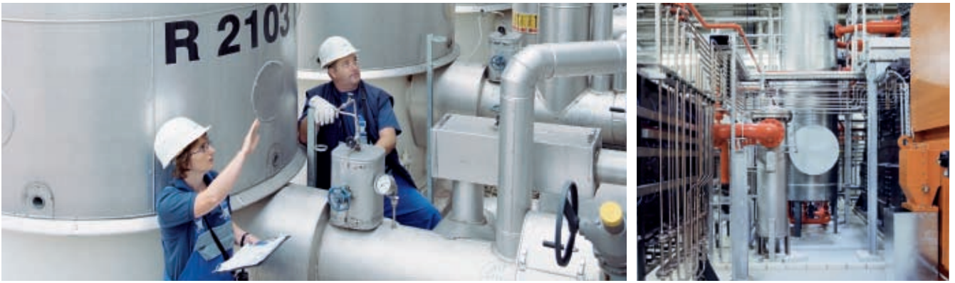
↳ Hydrogen liquefaction plant, Leuna, Germany
