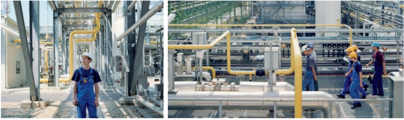
↳ Left and right: Kazincbarcika gas production plant, Hungary
